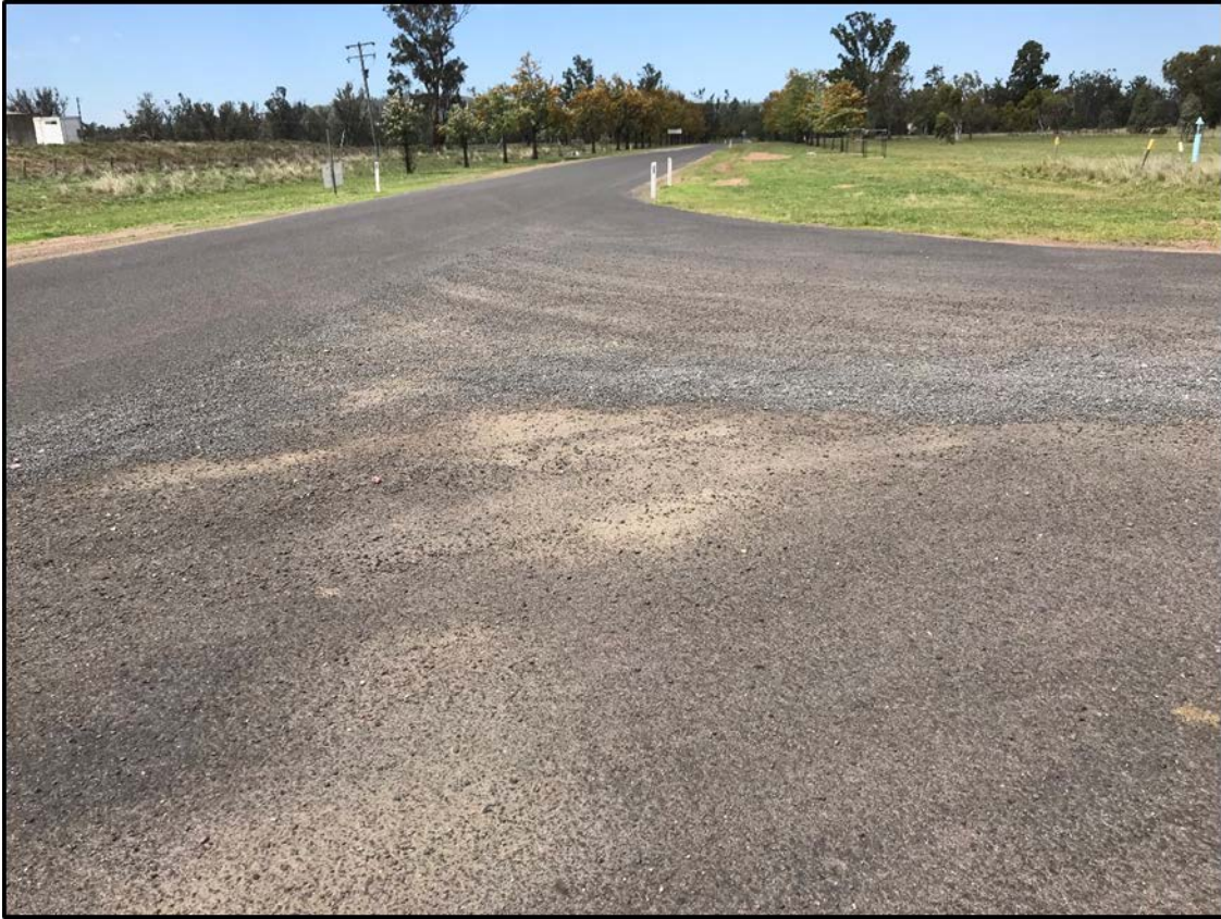
Photo 11 – View to right for driver exiting Old Blue Vale Road onto Kelvin Road
