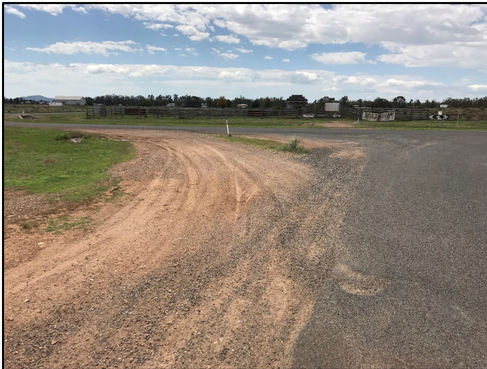
Photo 6 – View on Old Blue Vale Road at eastern end showing poor road maintenance at Kelvin Road intersection.
